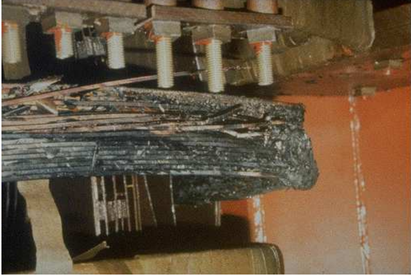
Extreme effect: New Jersey, March 1989: melted transformer
